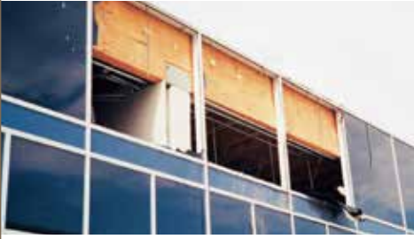
This glass wall facade was destroyed by high winds, leaving the building interior vulnerable to wind and rain damage.
