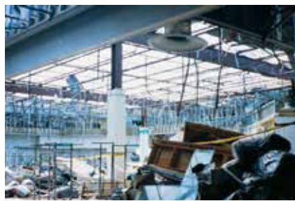
An insulated steel-deck roof was blown off this building.
