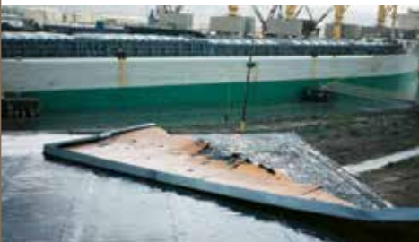
The damaged roof covering on this seaport building is mostly along the edge where wind forces are at a maximum.
