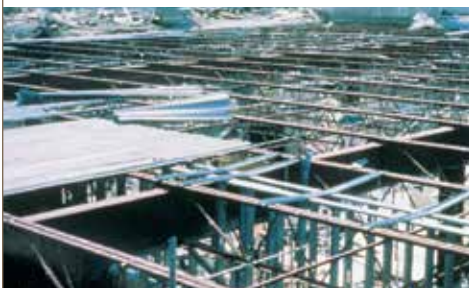
The lightweight concrete on this metal roof was severely damaged by a tropical storm.
